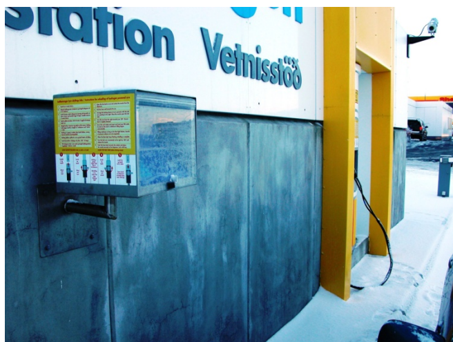
The hydrogen station with the card reader and surveillance camera
